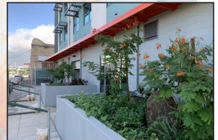
Completed Above-Grade Biofilters
