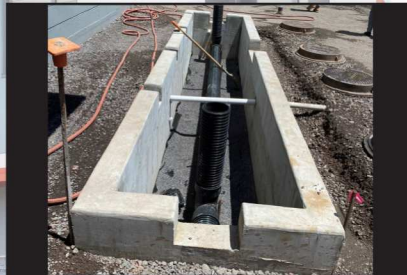
Construction on At-Grade Biofilter Curb walls and perforated drain pipes installed. Drain rock and engineered soil media to be installed next.
