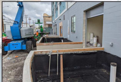
Construction of the Above-Grade Biofilters Planter walls are completed, and the waterproofing is installed. Drain rock and engineered soil media to be installed next.
