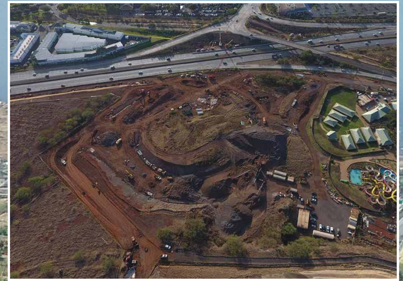
Mass grading of approximately 67,000 CY and 20,000 CY of embankment with grading of approximately 12 acres
