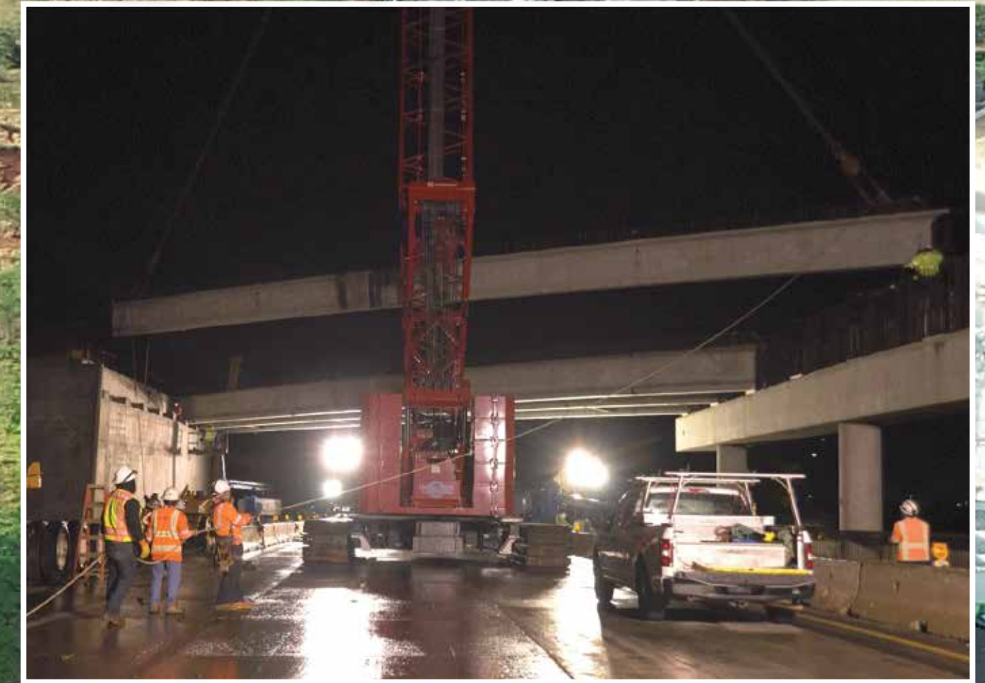
Wakea Overpass was constructed at night, requiring closure of H-1. Traffic detours provided to maintain access to Waianae Coast (H-1, facing eastbound).
