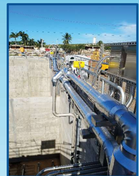
SAB Aeration Flow Control
