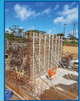
Step-Feed Aeration Basin
